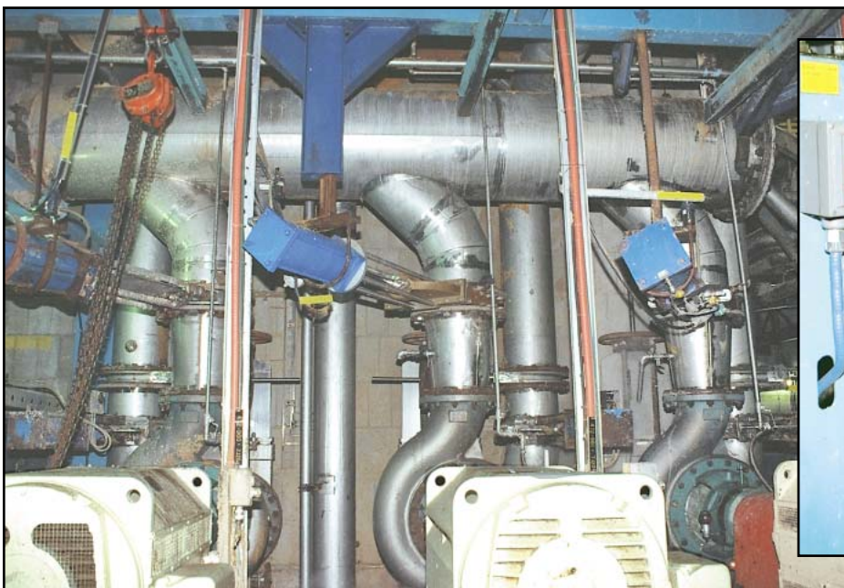
Multiple pump discharge isolation with pressure 70-90 psi (4.8-6.2 bar) white water.
