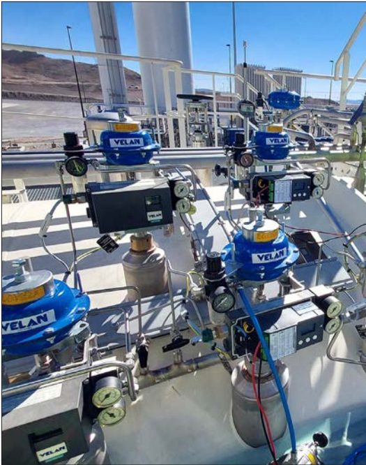
48 Cryogenic angle and straight regulating globe valves installed in a liquid hydrogen production plant located on the west coast of the United States and manufactured by Velan S.A.S., in France.
